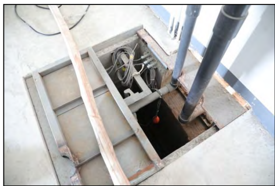
10#-11#后方含油污水集污池
